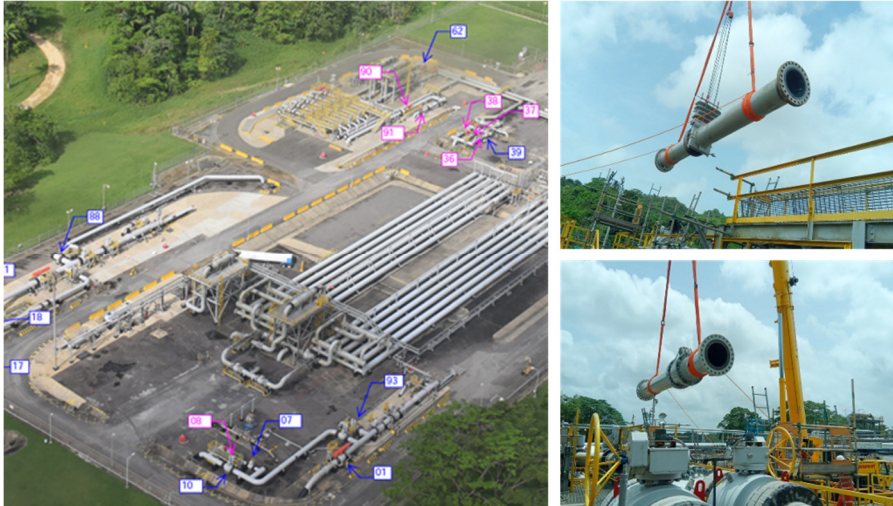
Left Image: Aerial view of BVU Facility Top Right Image: Removal of existing USM Meter Run Bottom Right Image: Replacement of USM Meter Run
